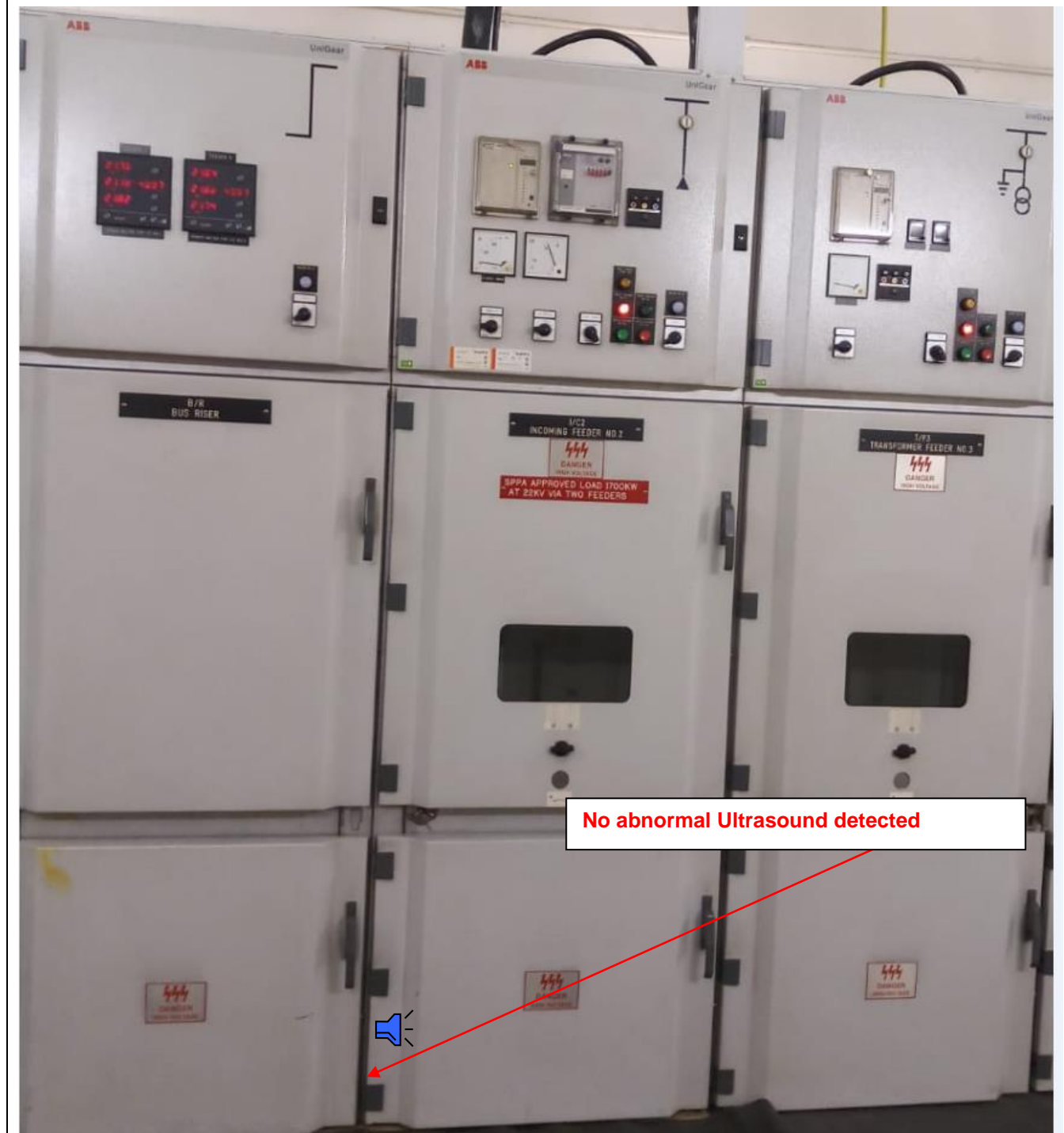
Phase Resolved Ultrasound Front Panel of "Incoming Feeder No.2" (Without VT) on 04 th September 2018
