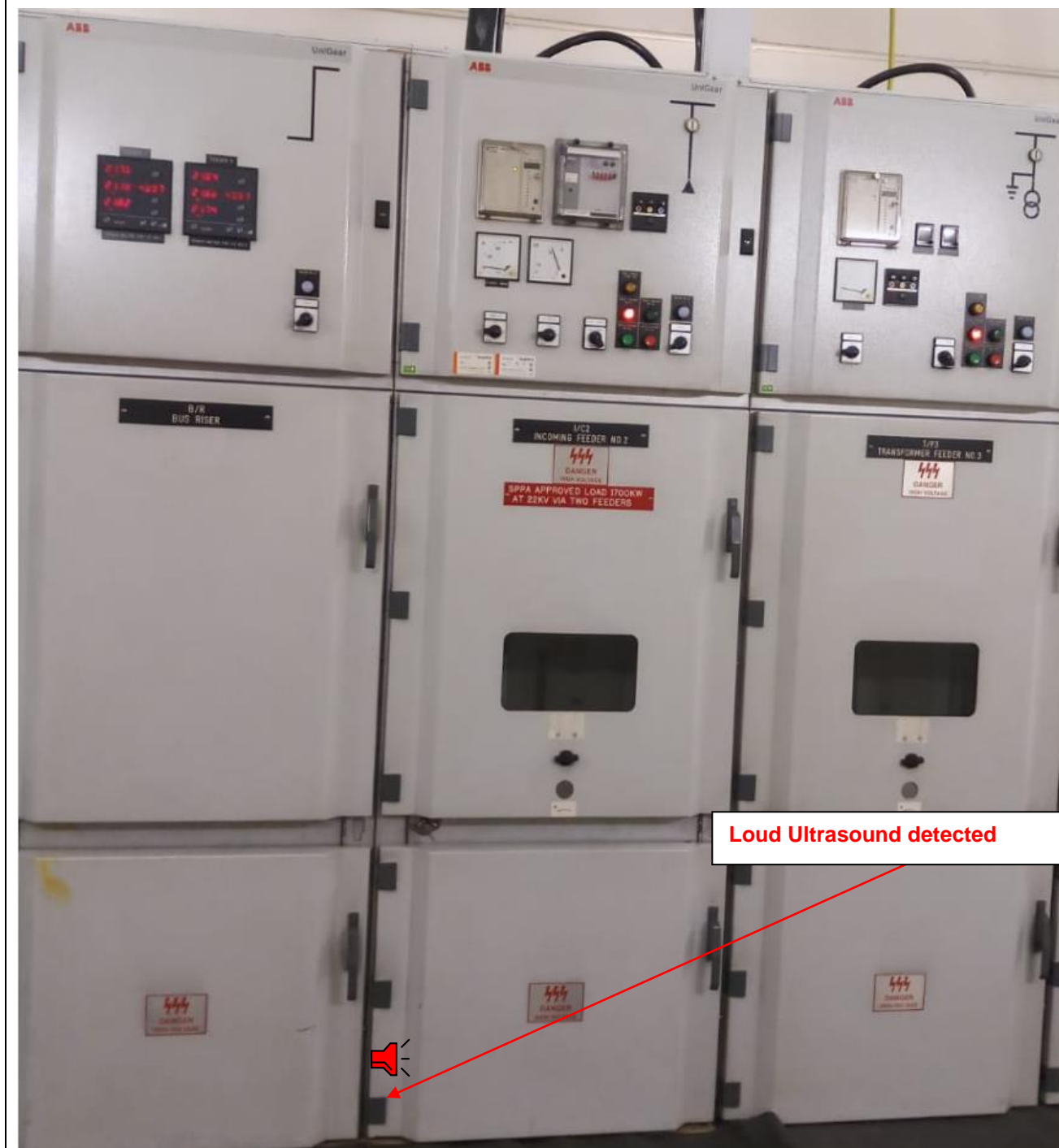
Phase Resolved Ultrasound on Front Panel of "Incoming Feeder No.2" (With VT) on 17 th August 2018
