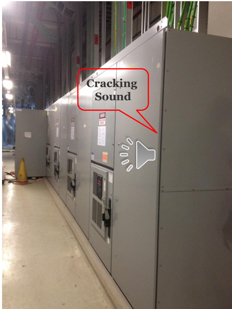
FRONT OF 6.6kV SWITCHGEAR
