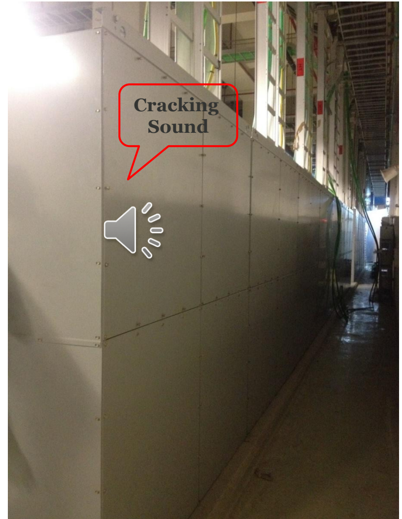
BACK OF 6.6kV SWITCHGEAR
